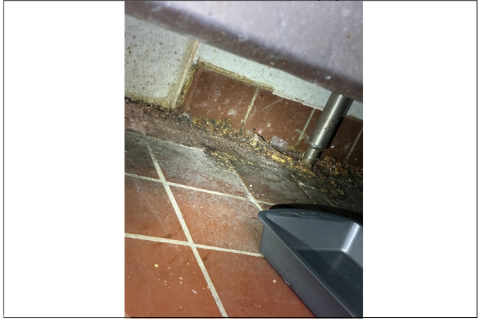
Soiled floors beneath equipment.
