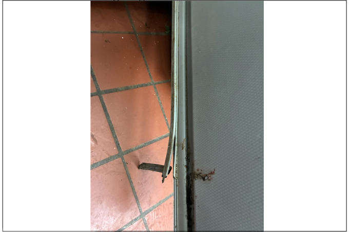
Damaged gasket on reach-in freezer.
